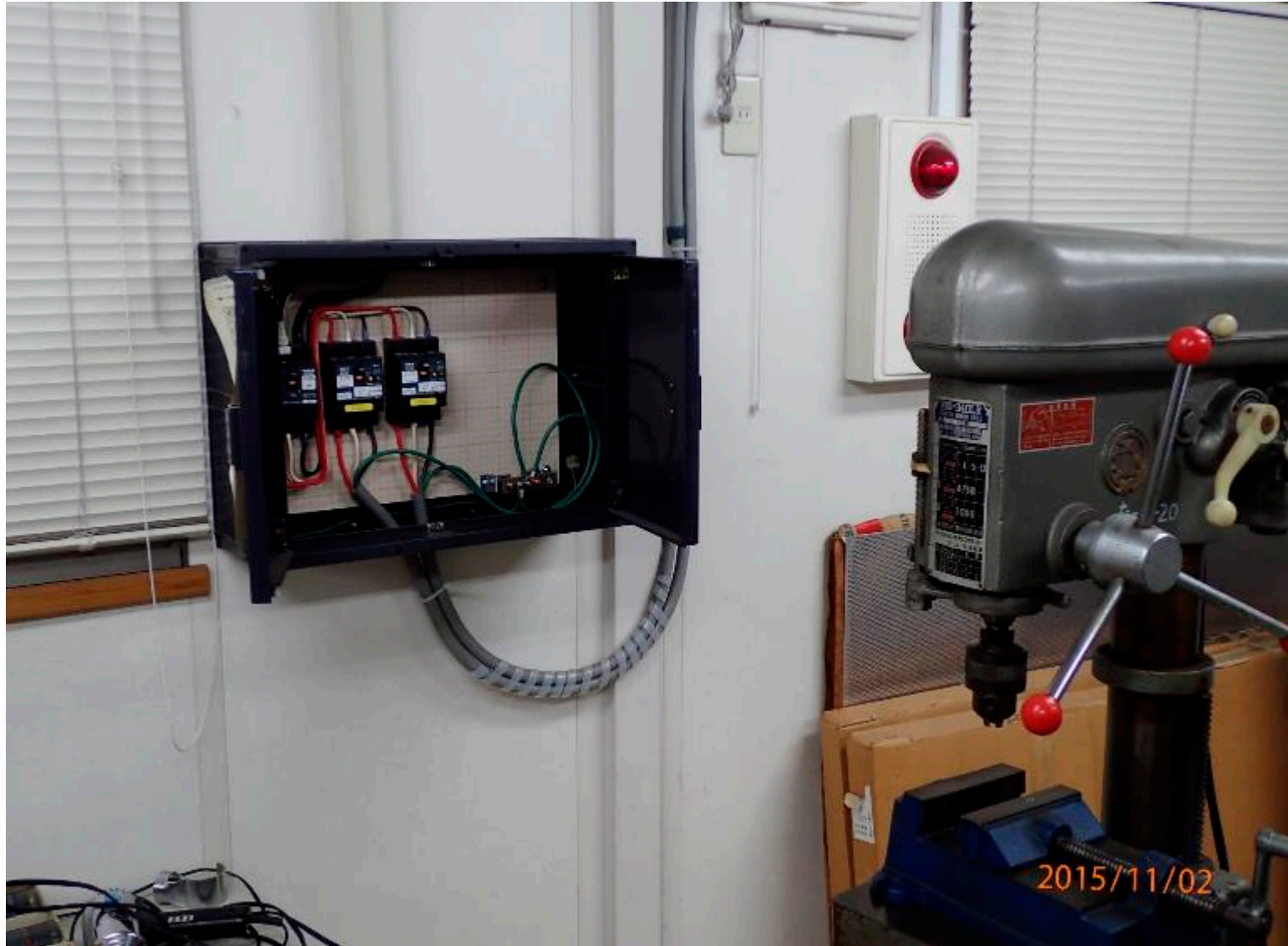
Figure 3 (a): Power distribution board in TAMA electronics shop
