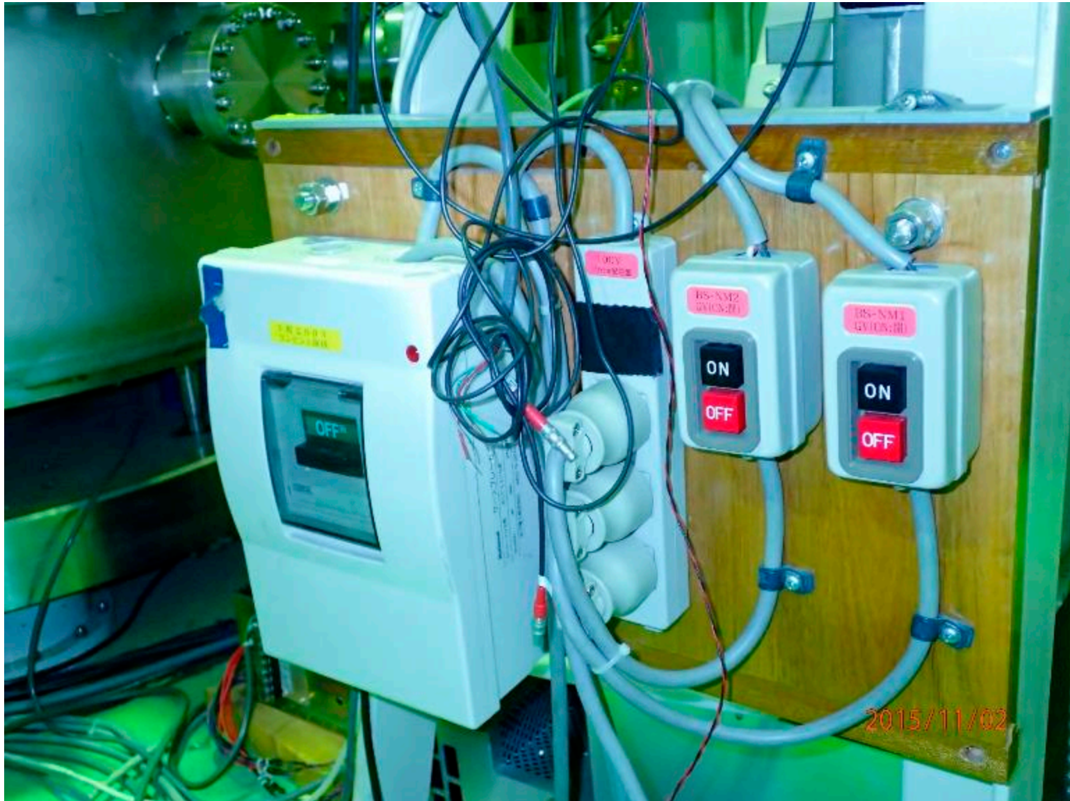
Figure 11: Operation panel for BS-NM1 and BS-NM2 Gate Valves
