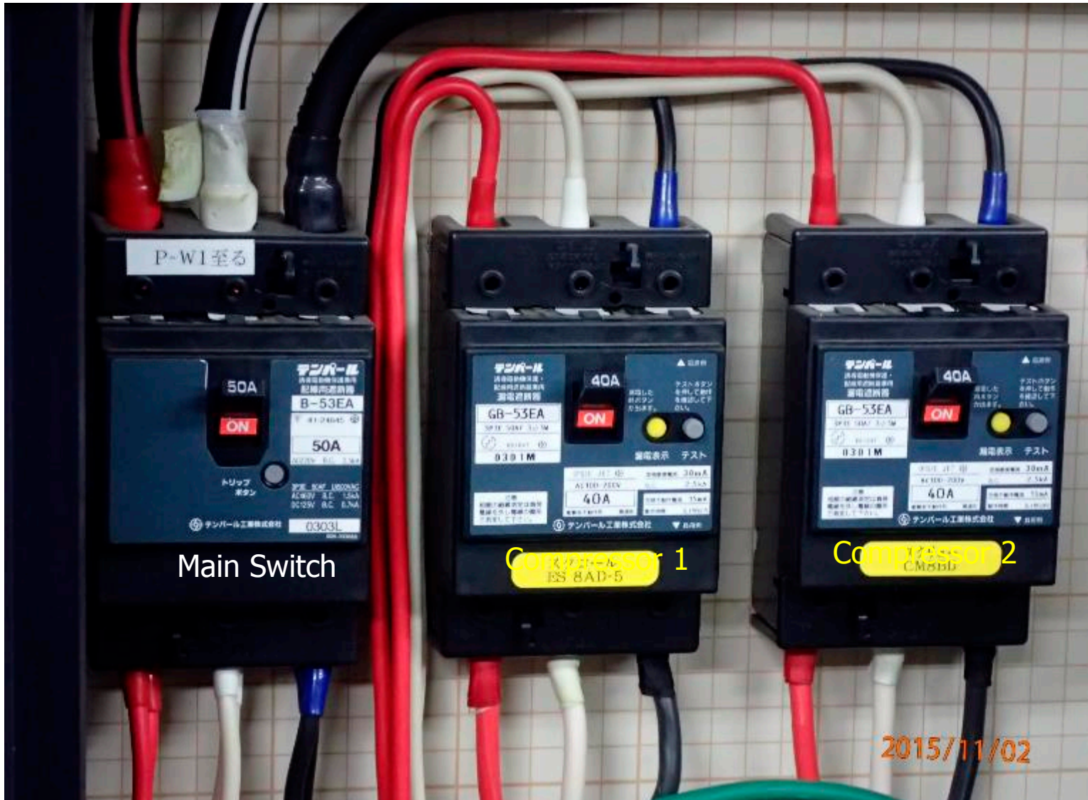
Figure 3 (b): Power distribution board in TAMA electronics shop
