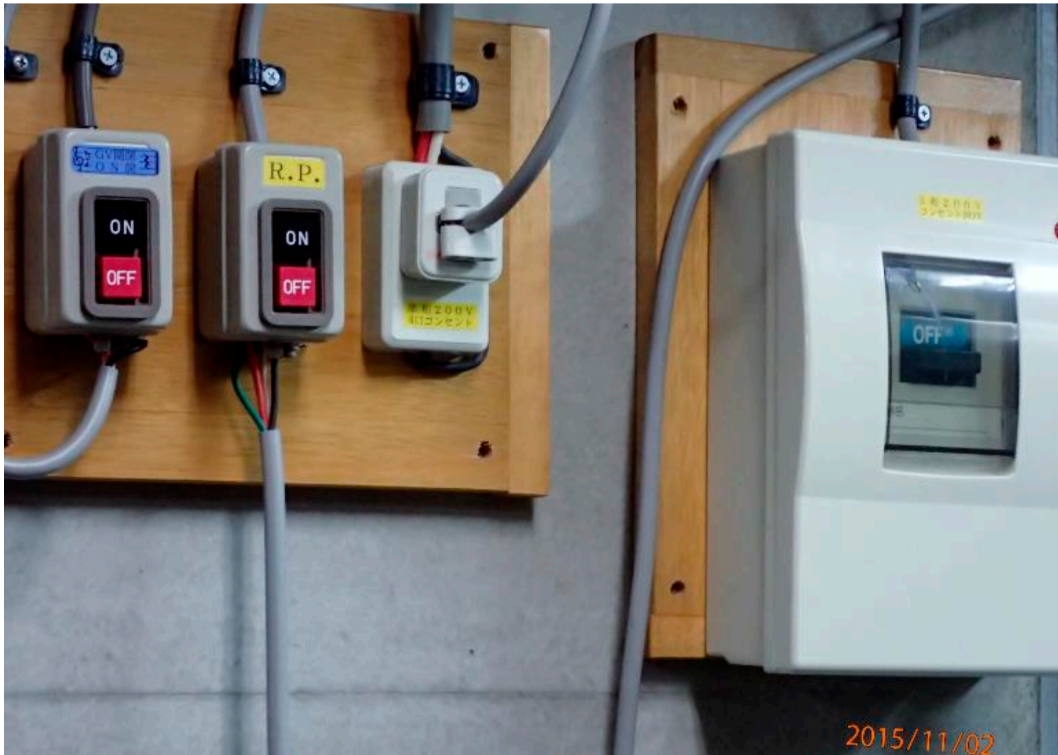
Figure 8: Operation panel for NM2 Gate Valve
